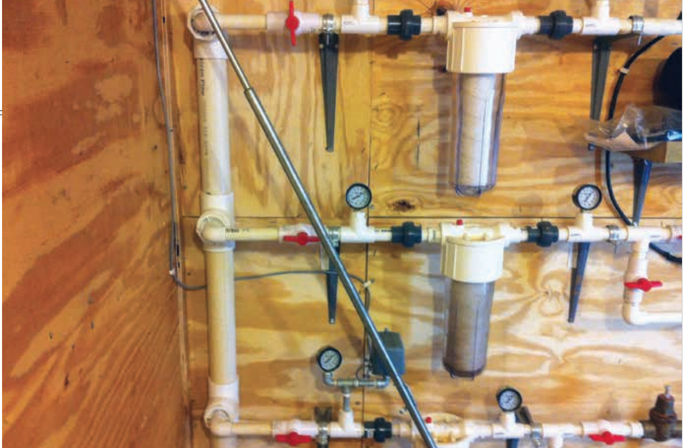
THIS SHOWS PROPER WATER SUPPLY LINE IN NEWER HOUSING. A 51MM PIPE IS USED TO SUPPLY ENOUGH VOLUME TO KEEP UP WITH DEMAND. SEPARATE 19MM PIPES, INDIVIDUALLY PROVIDE WATER FOR FRONT HALF DRINKERS, BACK HALF DRINKERS AND FOGGERS/COOL CELLS
