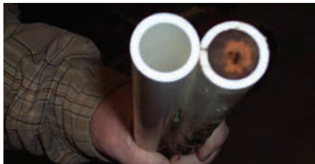
Biofilm (right) causing restricted water flow
